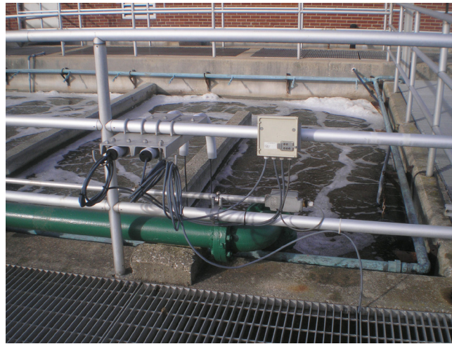
An IQ SensorNet module mounted tank side along with sensors for continuous process monitoring and control.
